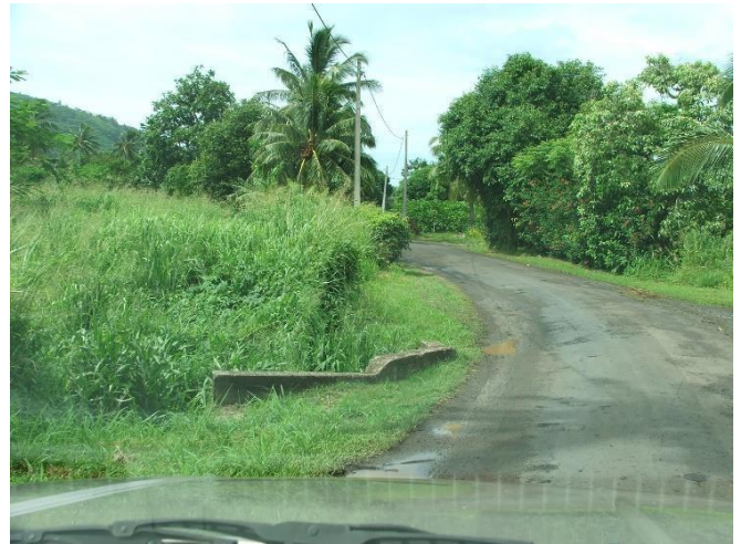
Overgrown weeds limiting visibility during day and night.
